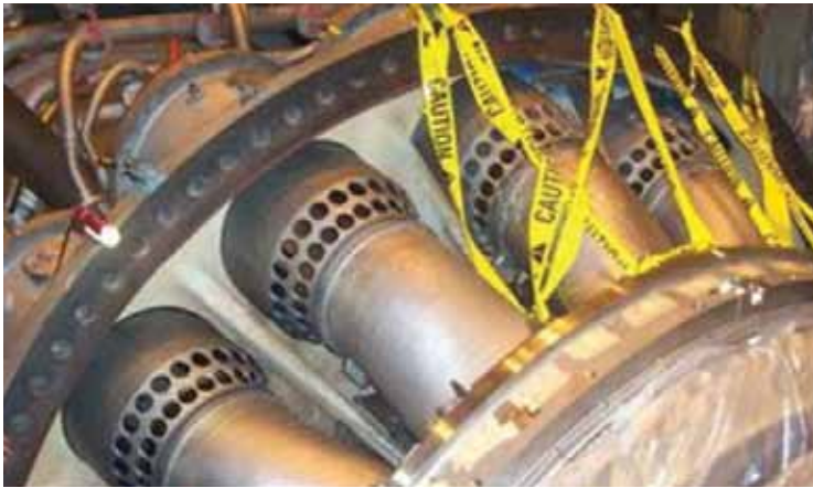
7FA-P1 Hardware Installation & Instrumentation
